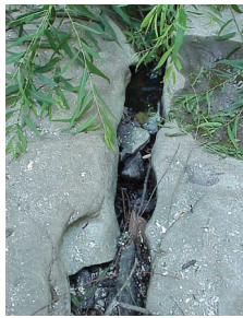
Water flowing through a crack in limestone at Gans Creek.
